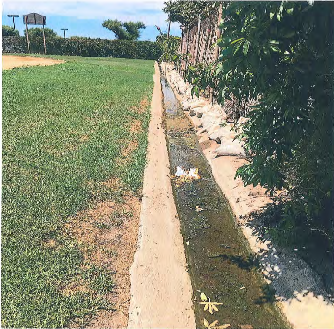
Rogers-Anderson Park East Property Line – Drainage Channel
